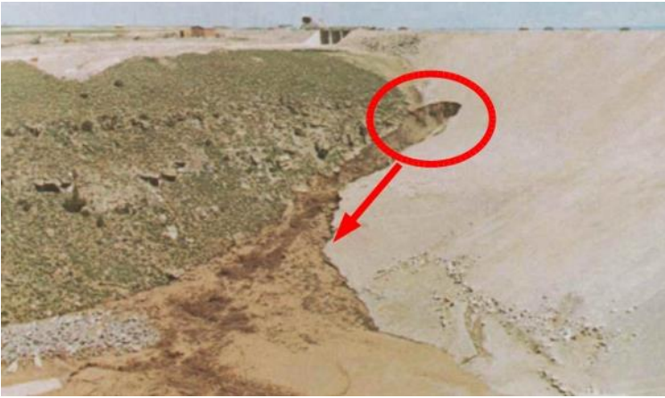
While keeping maintenance on the Teton Dam in Idaho, engineers noticed a small leak at approximately 7:30am, Sat, June 6th, 1976.
